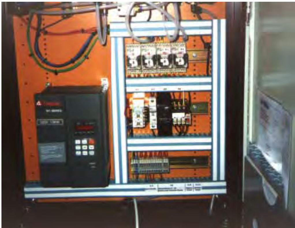
Electric box with frequency inverter
