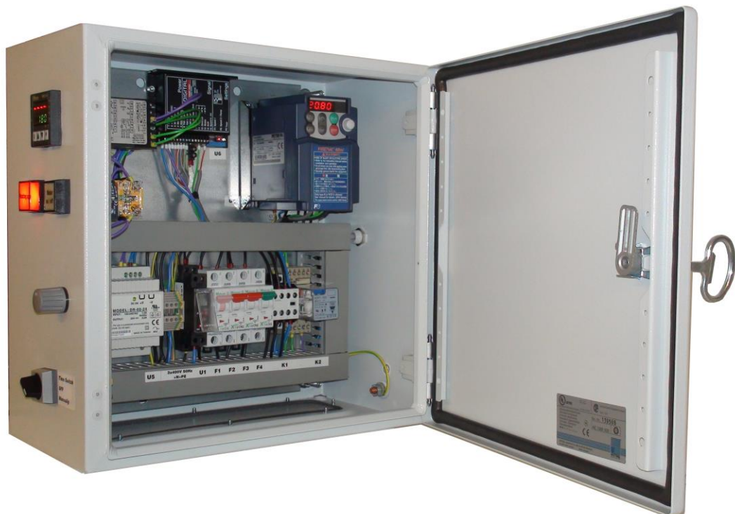
Electric Control Box for Hot Wheel Roll Coaters with motorized Backup Roll
